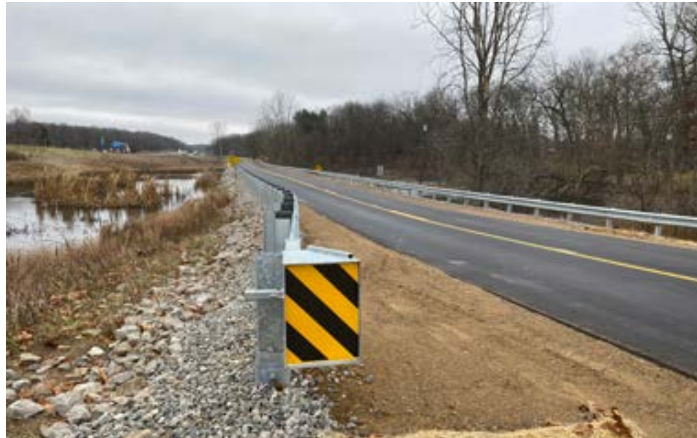
Final product of the aggregate lift performed on O Avenue between 4th Street and 6th Street.
