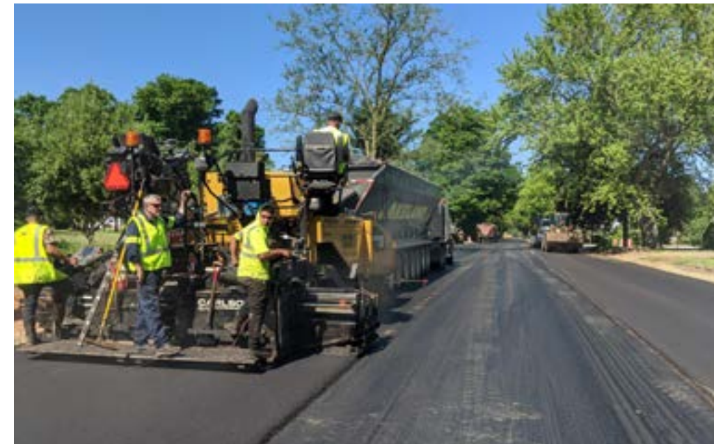
Top course paving on S Avenue between 34th Street and 36th Street.
