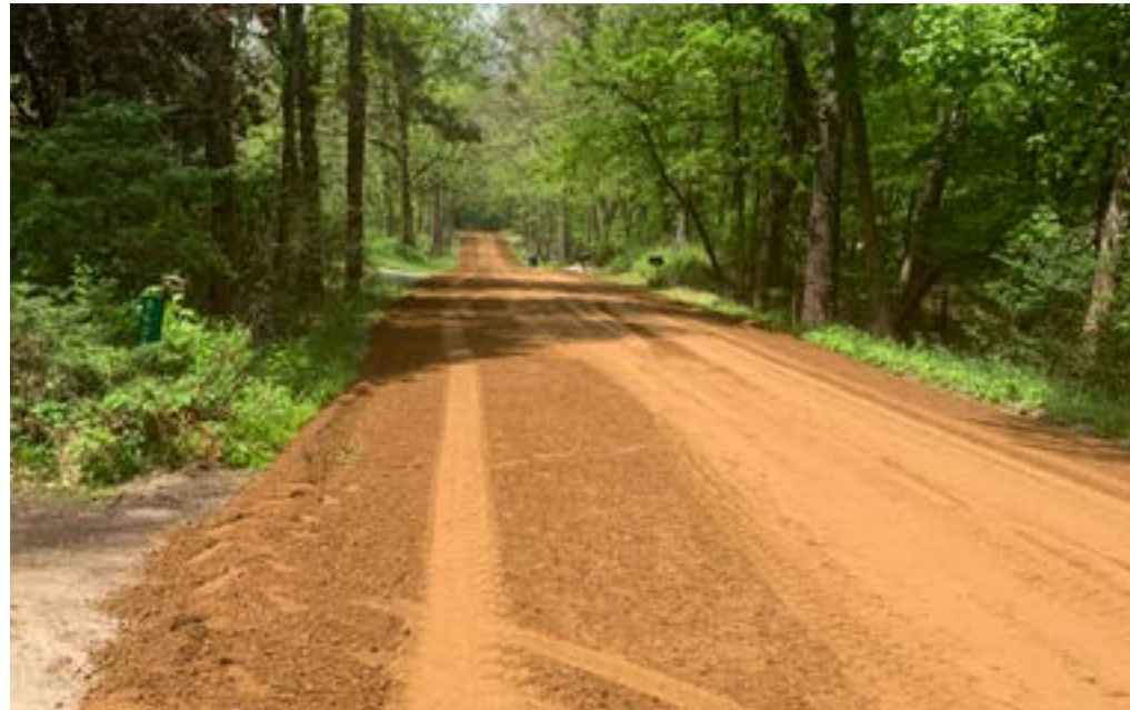
F Avenue with gravel and pulverization between 3rd Street and Far Hills Way - ready for the double chip seal!
